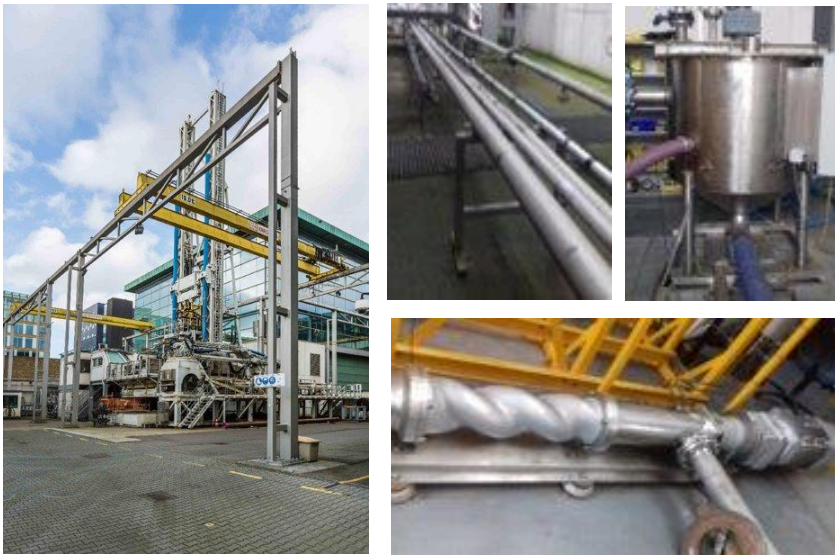
Flowloop installation, TNO Rijswijk
